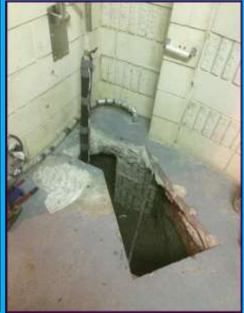
New PEX plumbing
